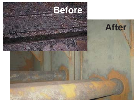
Coal tar Epoxy on a ballast tank in a ship before and after being stripped
